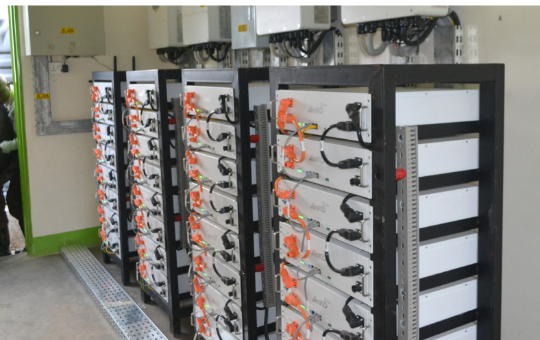
Nyakitokoli solar power plant control room fitted with solar batteries
